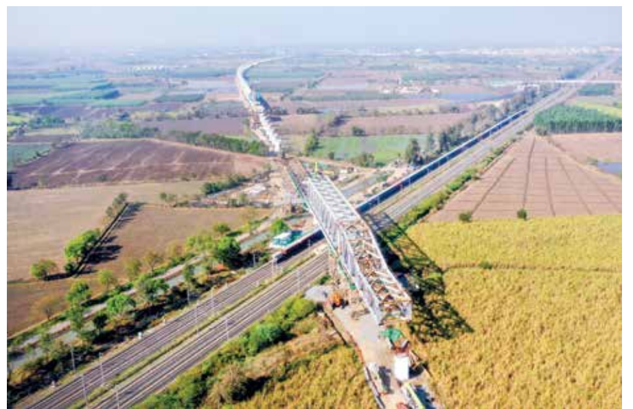
View of a 100m long and 14.3 m wide steel bridge built between Kim and Sayan for the Mumbai-Ahmedabad Bullet Train project in Surat, Gujarat.
