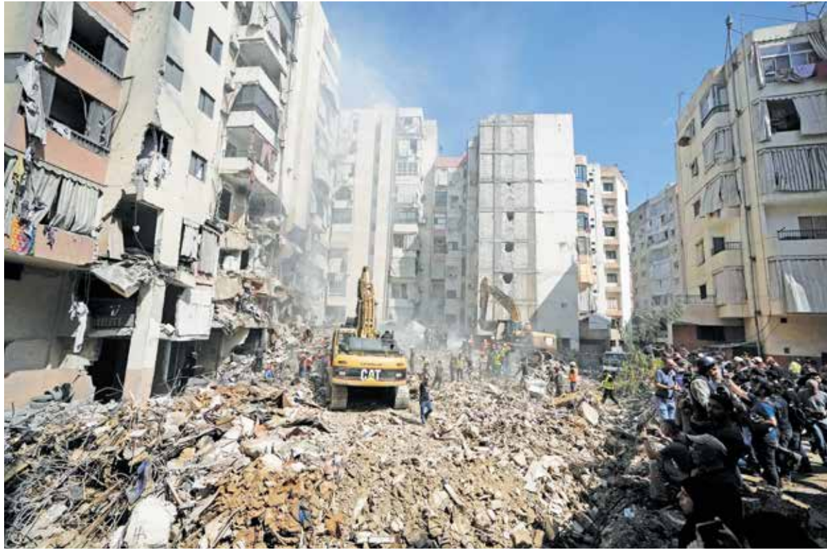
Emergency workers use excavators to clear the rubble at the site of Friday's Israeli strike in Beirut's southern suburbs on Saturday. Pic: APPTI
