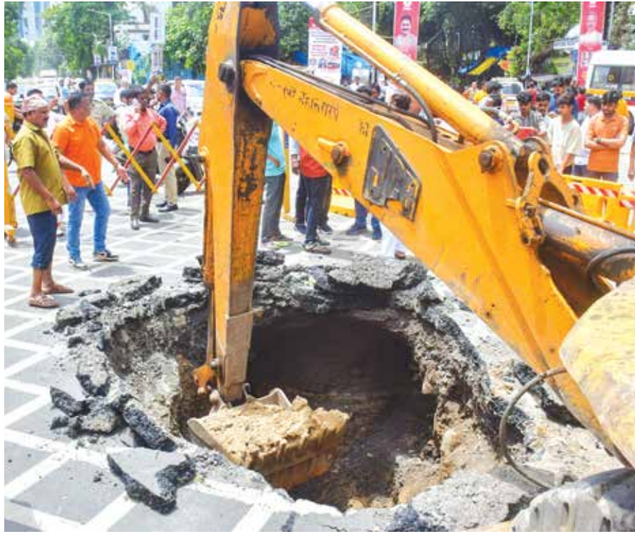
Repair work being carried out by Brihanmumbai Municipal Corporation (BMC) after a road caved in at Prabhadevi in Mumbai on Thursday. Pic: PTI
