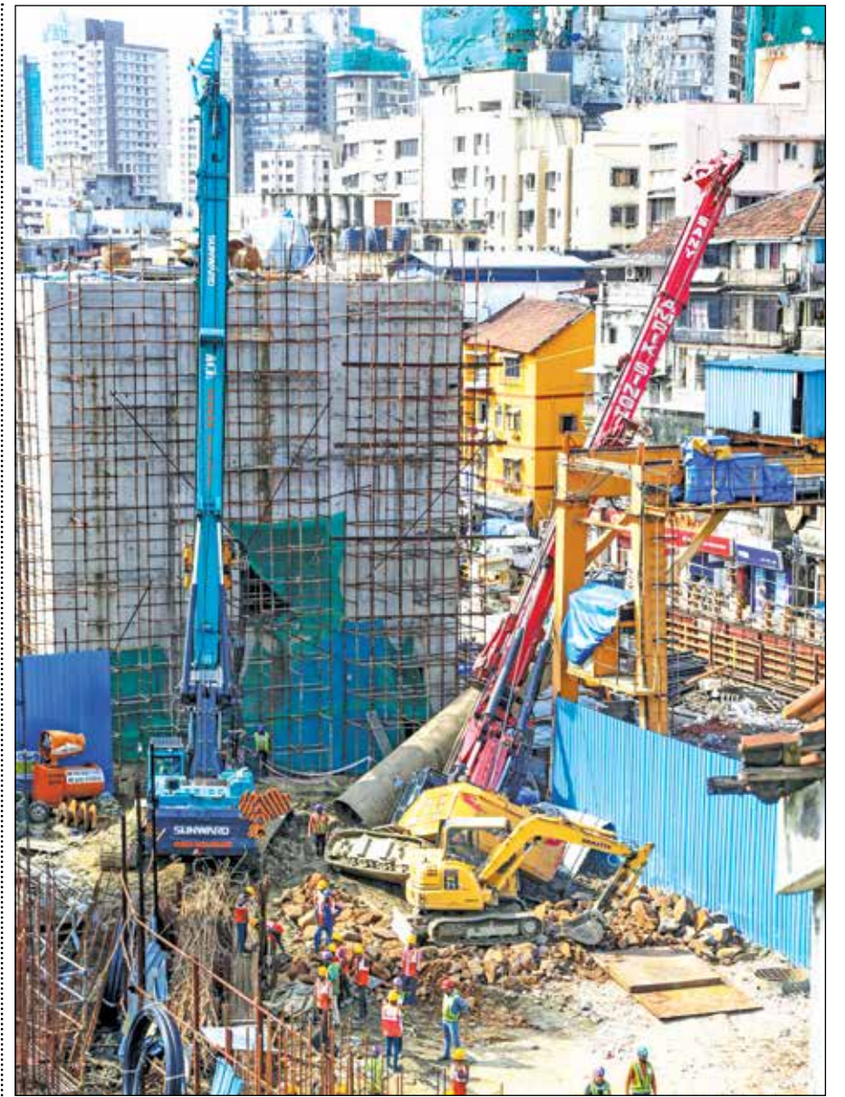
A crane toppled at the construction site of Mumbai Metro line 3, at Girgaon in Mumbai on Saturday.
